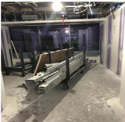
Pipe racks for miscellaneous studs
