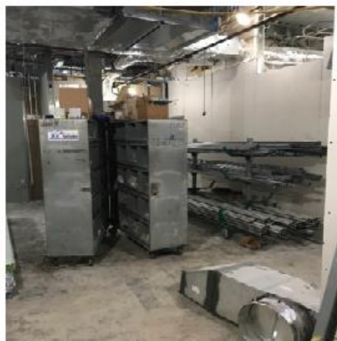
Pipe fitting stored in carts on wheels
